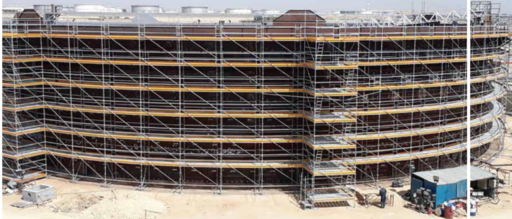
Circular tank scaffolded with a three-part side protection complete with system components
